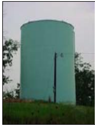
120,000 gallon Storage Tank located at Nolin Lake Estates
